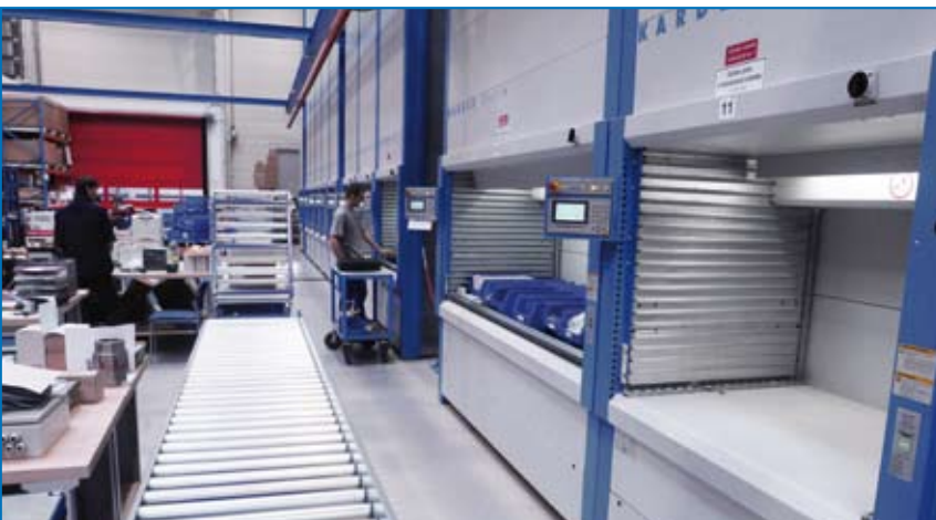
Automated storage systems have been complemented by conveyors for maximum picking convenience.
